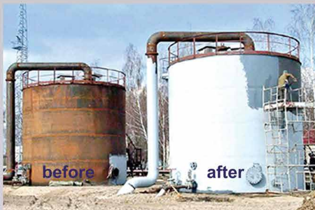
Kobrin Oil Pumping Station Belarus
