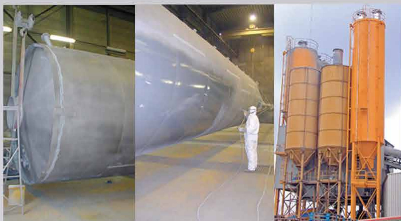
Storage tanks Paesen Concrete Mill Belgium
